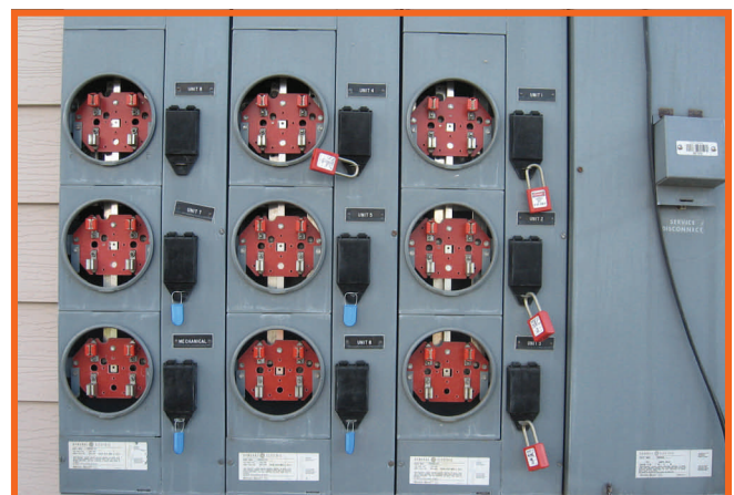
FWA demo utilities at building 4223 has a scheduled completion date of May 31.
