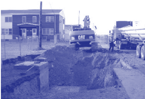
Construction employees replace a water main associated with the 3rd Street project.
